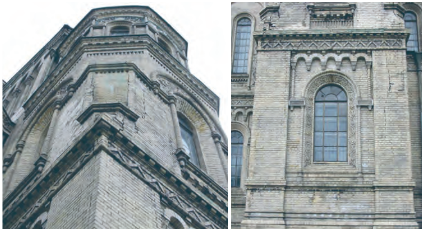
Defects caused by penetration of atmospheric humidity and freezing of the brickwork.
