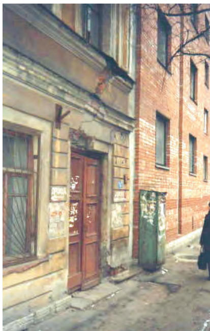
Classical settlement related cracks which appeared in a house adjacent to a new building with wrongly constructed foundations. The new house (in this picture located on the right) developed settlements and "pulled" its neighbor into the trough. Below you see the settlement diagram (mm)
