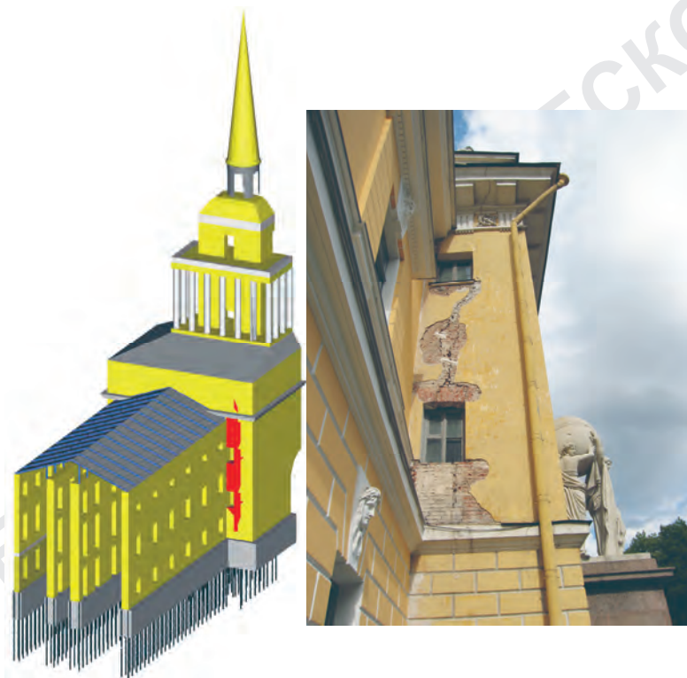
The figure on the left indicates the zones of possible development of inclined cracks, according to the calculations; the photo on the right shows the actual development of cracks on the Admiralty building.
