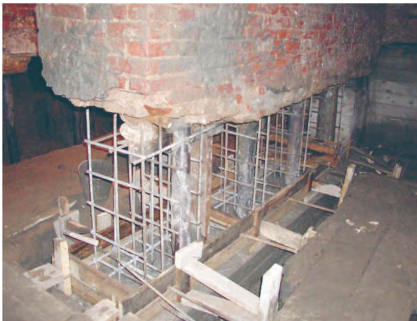
All walls of the retaining structure got suspended on thin strengthening piles. It was possible to look at the undercut of the foundation footing.
