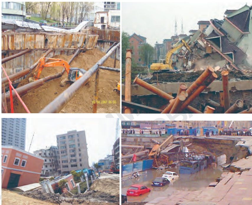
Examples of pit failures in various cities.
