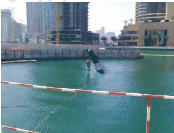
Infinity Tower pit collapse, Dubai (2007).
