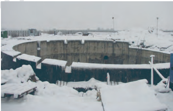
Sunk shaft of a sewer pump station (appearance following the underpinning with bored piles and the onset of tilt up to 1200 mm).
